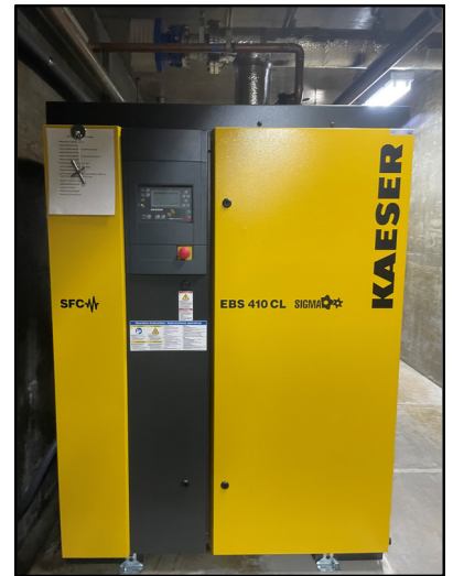
New Kaeser blower unit
