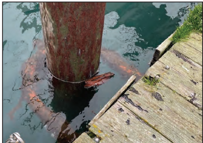
Low freeboard resulting in submerged pile collar.
