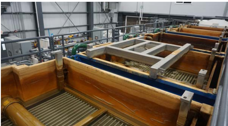
Membrane Filters at Water Treatment Facility
