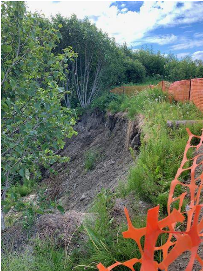
Hornaday Park slope failure
