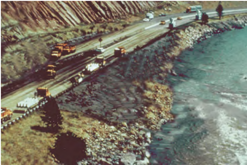
A rainstorm-generated debris flow a couple of months after a wildfire, adjacent to the Colorado River near Glenwood Springs, Colorado, caused major interstate traffic disruption in September 1994.
