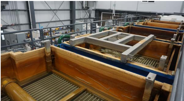
Membrane Filters at Water Treatment Facility
